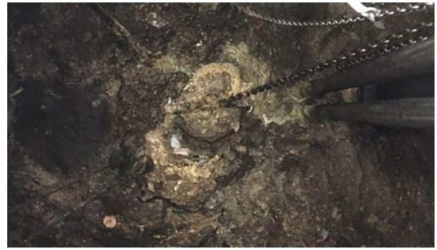
Figure 1. Lift station highly impacted by wastewater FOG loadings. Accumulated grease requires frequent removal and disposal.
